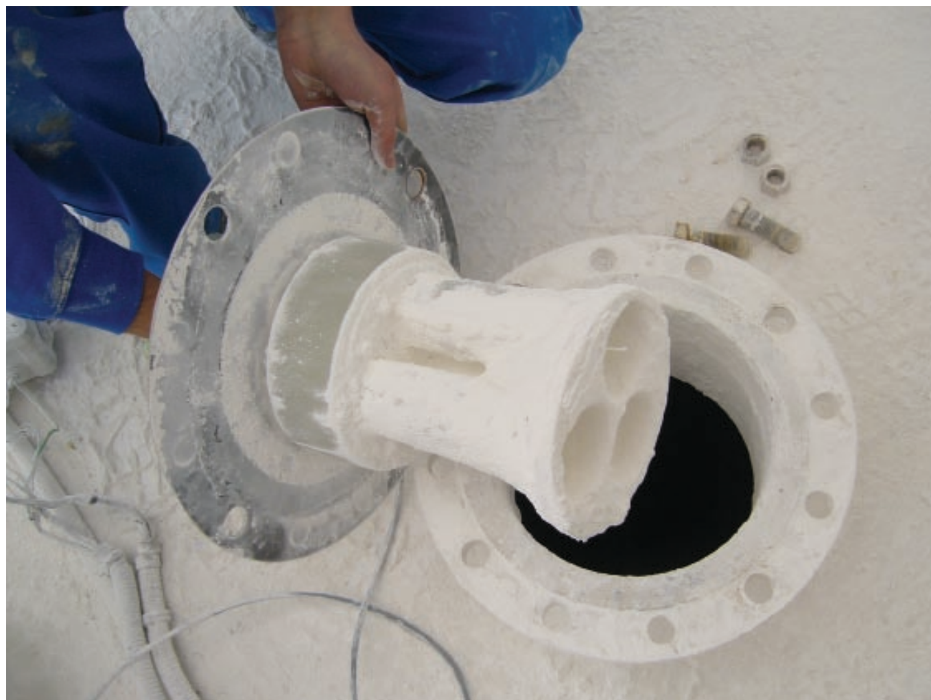
Figure 3 - Acoustic sensor transducer after one year of service in calcium carbonate (photo courtesy APM Automation Solutions Ltd)
